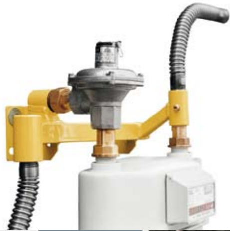
Gas meter connection hoses
